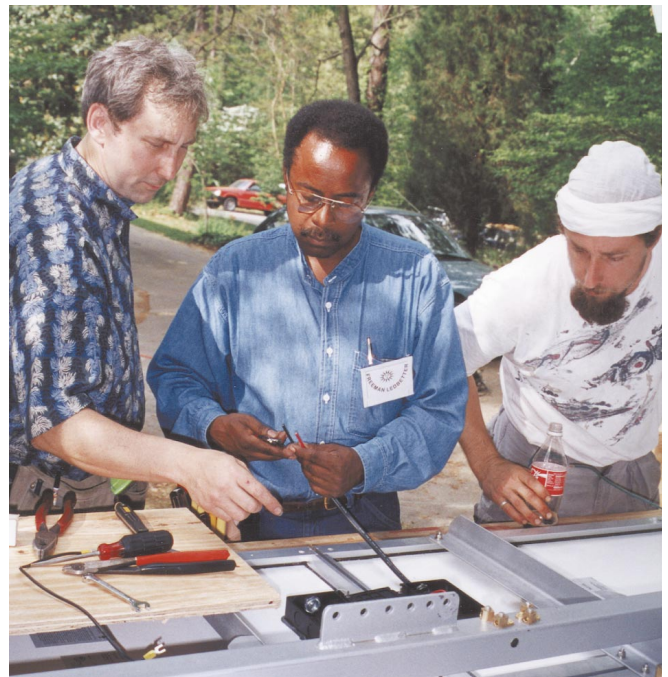
Above: Chris Carter of Solar Village Institute teaches the class how to properly mount and wire the photovoltaic array. Since PVs will easily produce power for over ten years, details such as module wiring are critical if the array is operate for ten years without problems.
